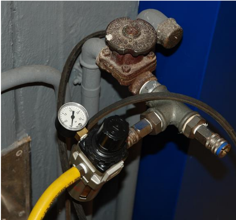
Fig. D.2. Inlet pressure regulator, number 1 in fig. D.1
